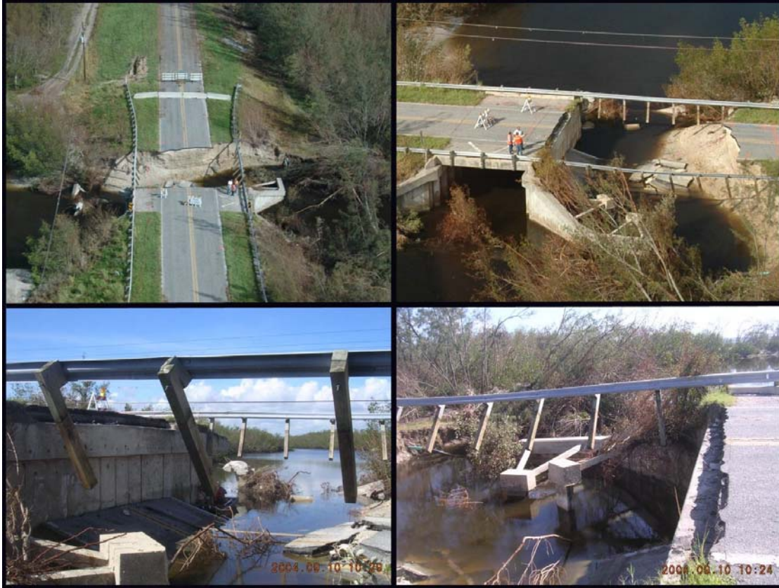
Photo 29: U.S. Highway A1A Breakthrough at Little Mud Creek (R69.5)
