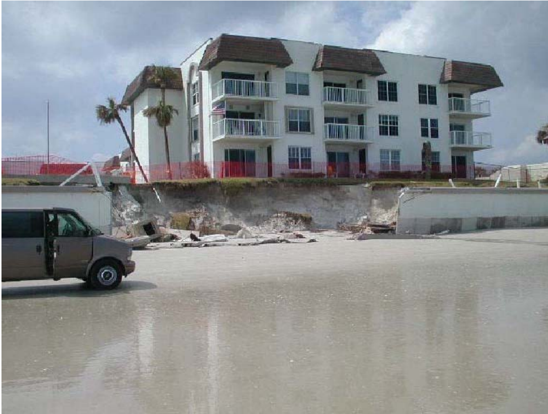
Photo 4: Seawall Damage, New Smyrna Beach
